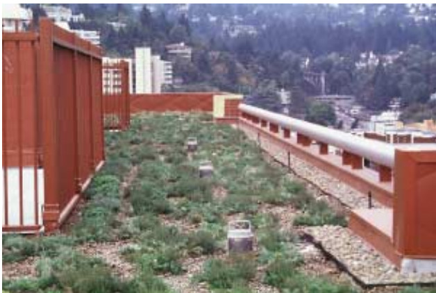
Hamilton Apartment Building Green Roof, Portland, Oregon
