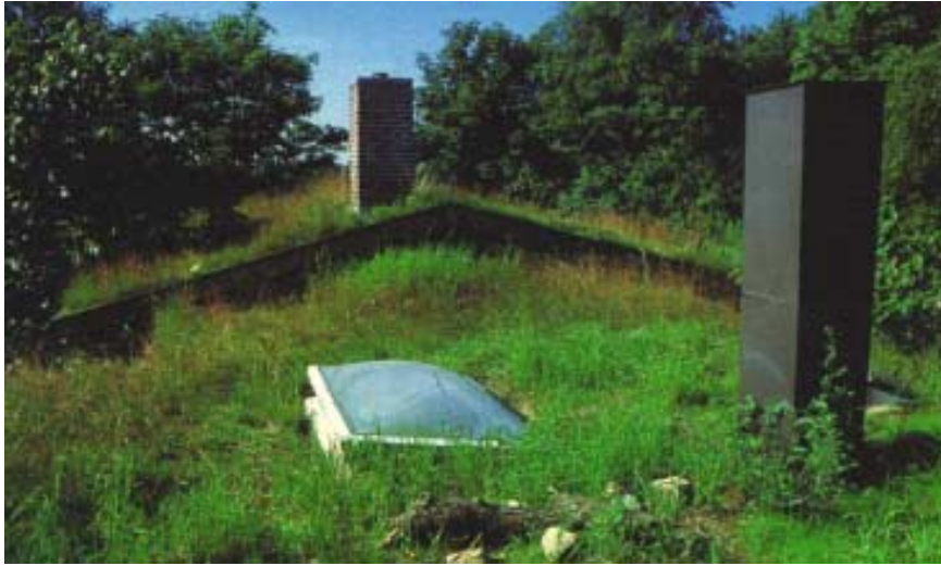
Green Roof on a Sloped Roof of a House in Northern Germany
